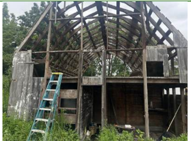
Photo 4 - View of the smaller dilapidated barn on the site
