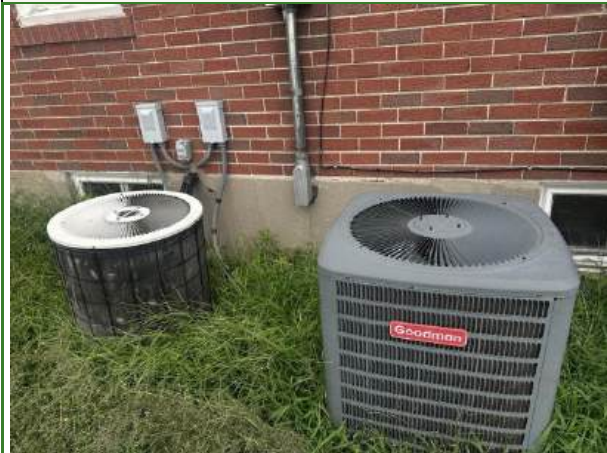
Photo 9 - View of the outdoor ac units on the site
